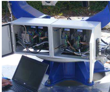
View to controller boxed for the drive engines (four axes)
