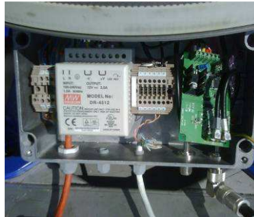
a) Tx and Rx connector board with LNB DC control ...
